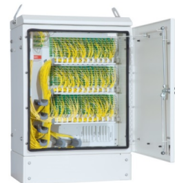
Fiber Distribution Hub
