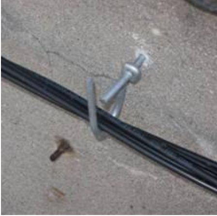
D Rings for Horizontal Cable Storage
