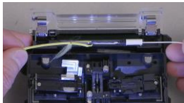
22. When the splicer beeps, the shrink process is complete. Confirm complete shrinkage of the protection sleeve.
